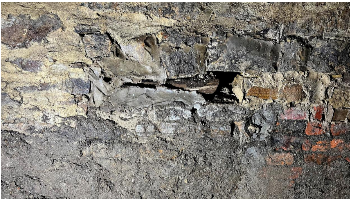
End of flue in boiler room.
